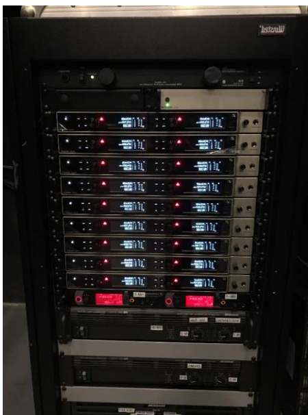
One of the Sennheiser racks at WKAQ
